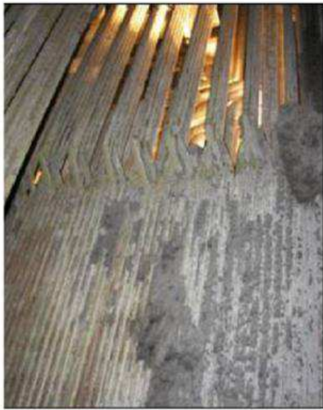
Screen tubes BEFORE operation
