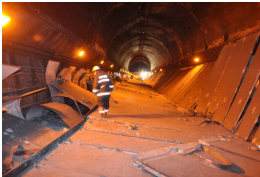
Fig. 1.6 Sasago Tunnel Accident by loose bolt 24)
